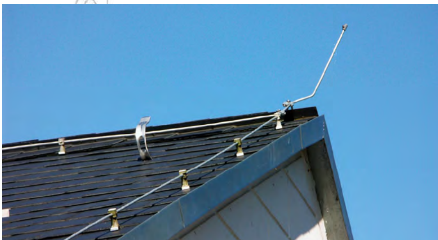
Figure 2.16 A lightning conductor will conduct electric charge from lightning safely away from a building to the earth.
